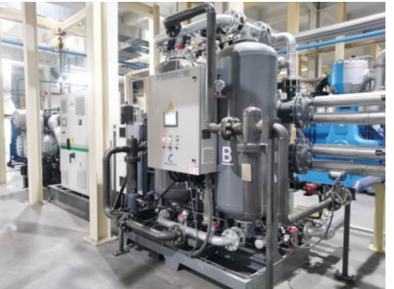
Project Client Food Industry Machine Model 4 × 45 m³/min Zero-Air-Loss Blower-Heated Regenerative Adsorption Dryers (40 bar)
