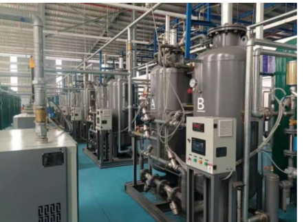
Project Client Overseas Market Machine Model 5 Refrigerated Air Dryers + Nitrogen Generators
