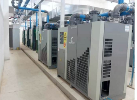
Project Client Advanced Materials Industry Machine Model 5 × 55 m³/min AH Series Refrigerated Air Dryers
