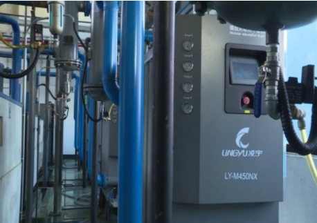
Project Client A Foreign-Invested Electromechanical Company Machine Model 50 × 50 m³/min Modular Adsorption Dryers
