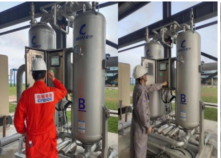
Project Client Petrochemical Industry Machine Model 4 × 40 m³/min CCS-Certified Adsorption Dryers
