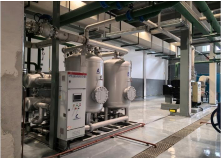
Project Client Pharmaceutical Industry Machine Model 3 × 85 m³/min Zero-Air-Loss Blower-Heated Regenerative Adsorption Dryers
