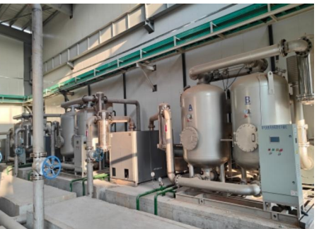
Project Client New Energy Materials Machine Model 9 × 200 m³/min Blower-Heated Regenerative Adsorption Dryers
