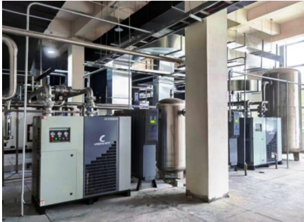
Project Client Pharmaceutical Co., Ltd. Machine Model 4 × 28.5 m³/min Refrigerated Air Dryers + Modular Adsorption Dryers
