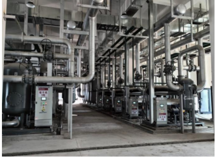
Project Client New Energy Industry Machine Model 5 Sets of Zero-Air-Loss Blower-Heated Regenerative Adsorption Dryers + Refrigerated Air Dryers
